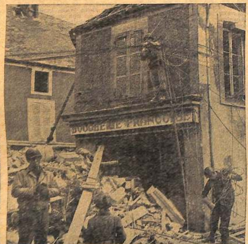
U.S. Army Signal Corps Photo SIGNAL CORPS men string wires in shattered French town. They kept lines open under withering fire, played vital role in D-Day operation of famous infantry regiment. (See story above.)
