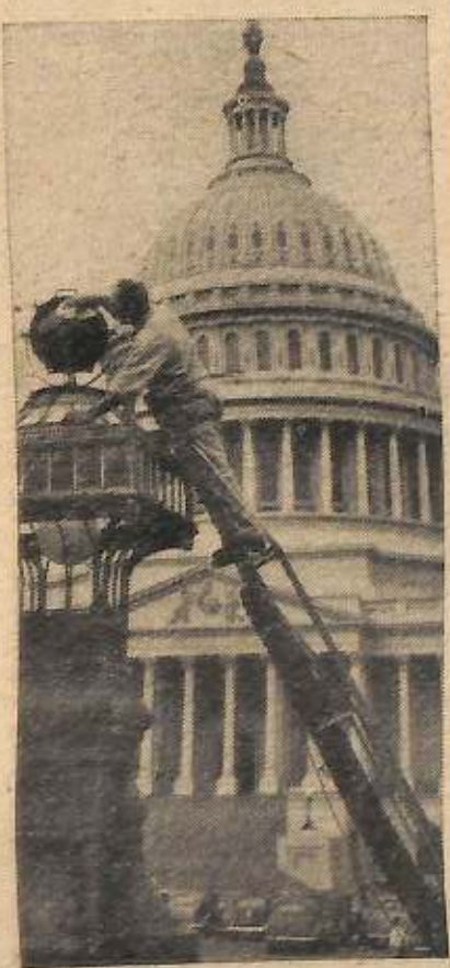
WHEN THE LIGHTS go on again, once hostilities in Europe end, no place will shine brighter in the U.S. than the nation's Capitol building, dimmed since "the day of infamy." Workmen are shown rushing (and we're hoping they're not too optimistic) the cleaning of the huge floodlights which will brighten up America's number one building.
